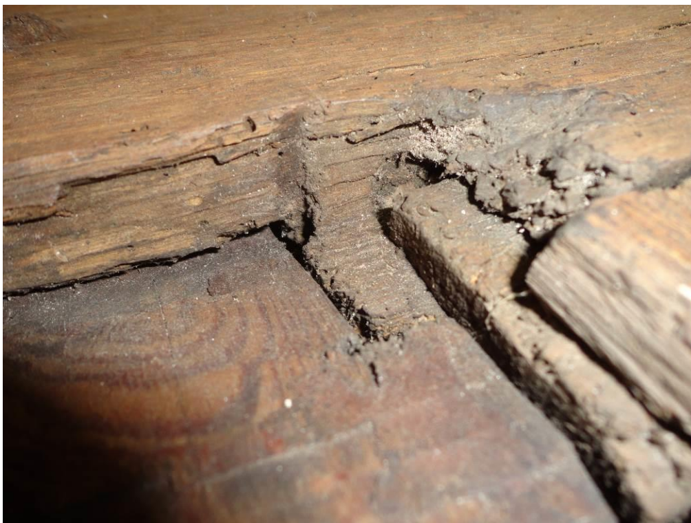
Figure 5: Stopped loose tongue groove at the top of board 2 with loose tongue (DM)
