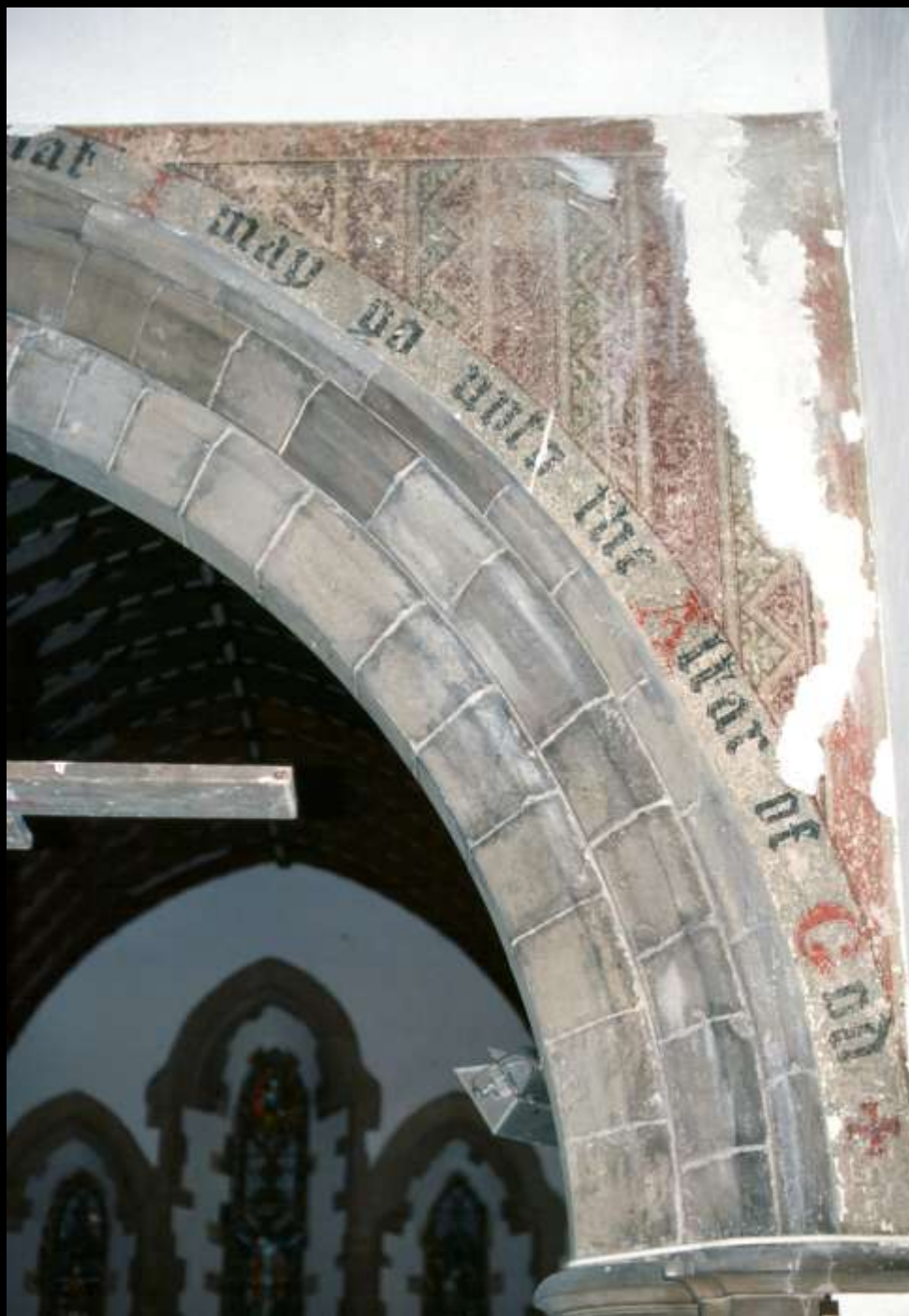
Caunton: C19th texts and stencil decoration on chancel arch. Uncovered during repair work.
