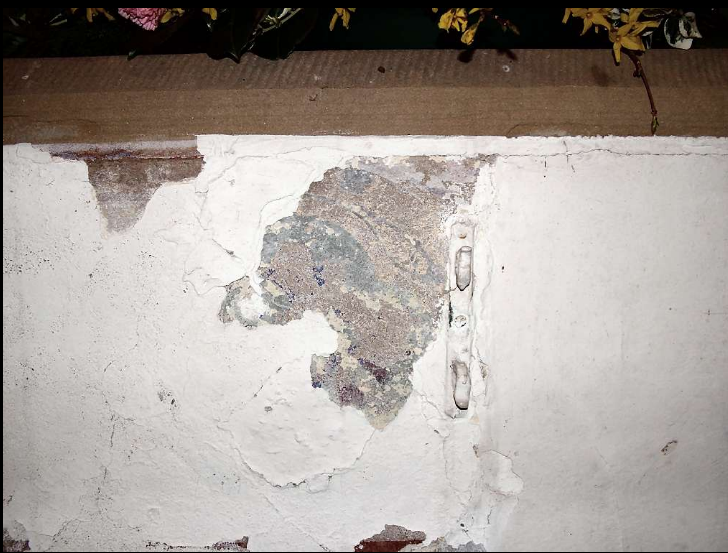
Hockerton: decorative paint traces visible under flaking overpainting
