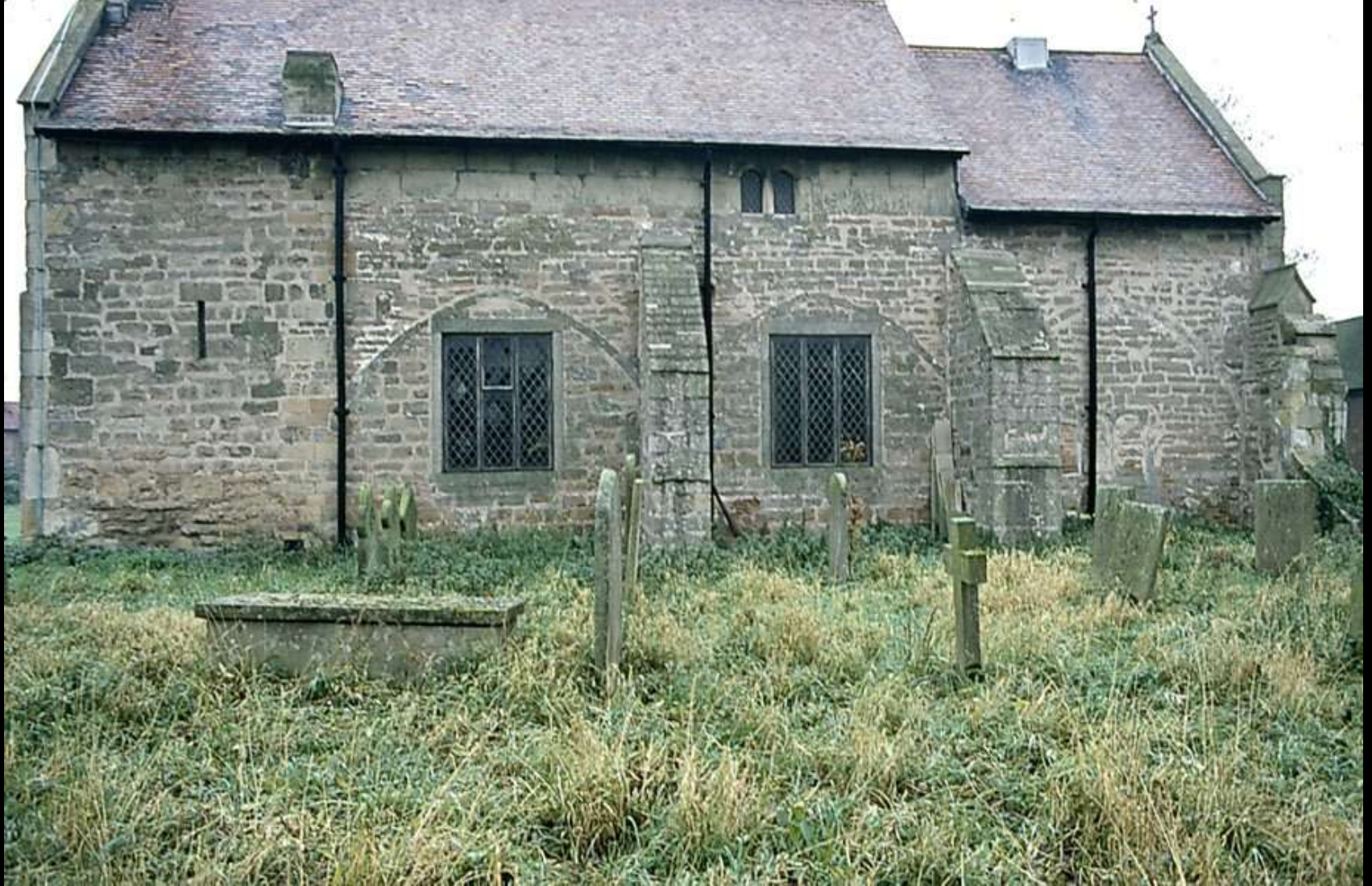
Complex fabric alterations at Edingley, St Giles, Notts. Including blocked S. aisle arcade, and S. chancel chapel arcade
