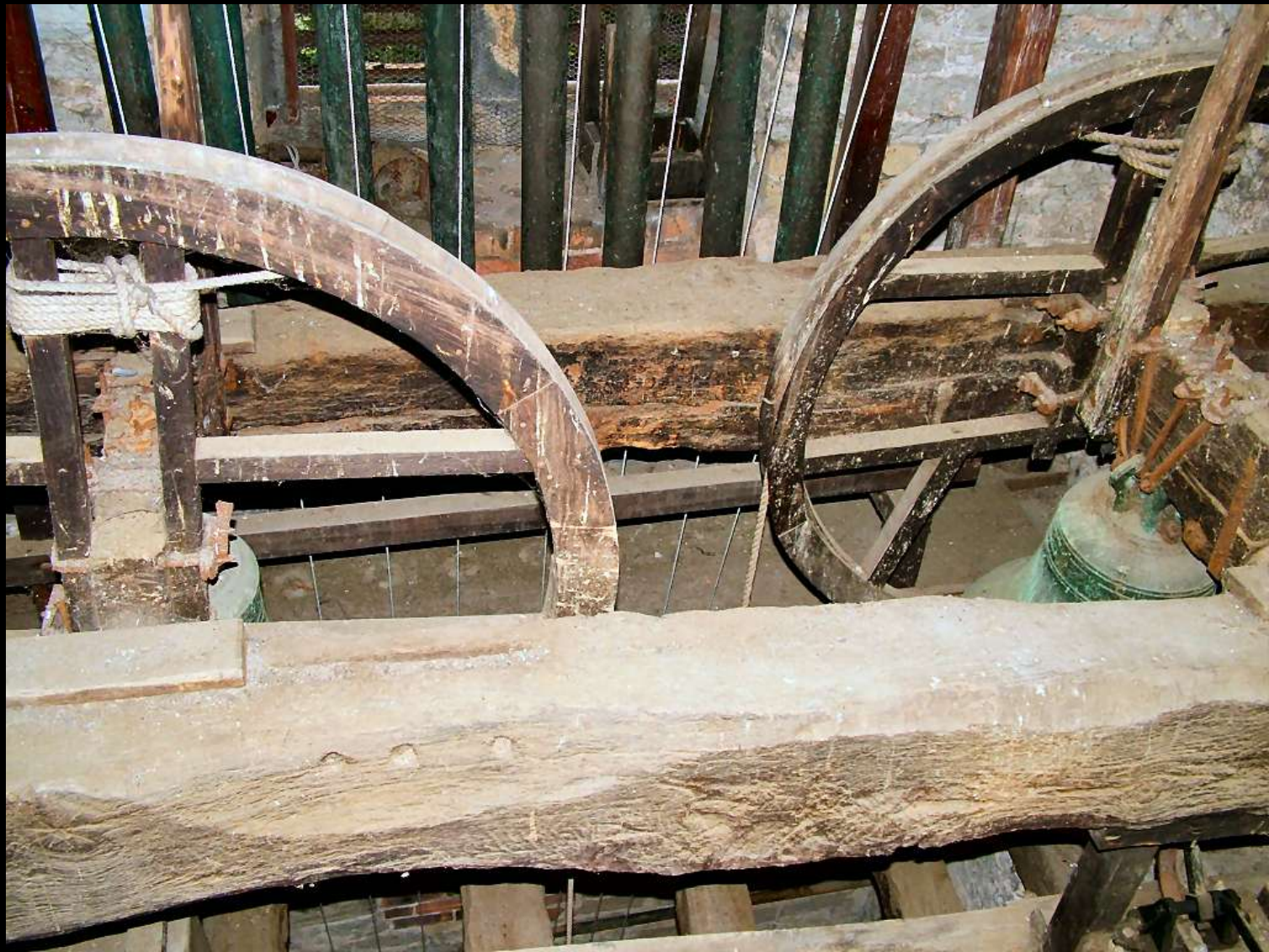
Bleasby. Simple Elphick 'B' frame suspended between belfry window cills. Tree-ring dated to AD 1476
