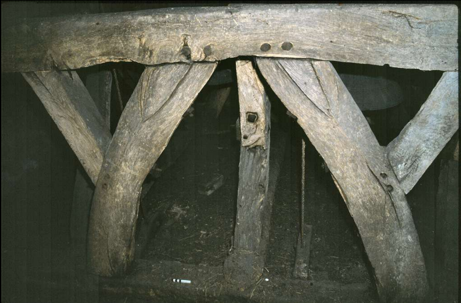
Fledborough: early form of Elphick 'V' frame with curved braces. Undated but probably late medieval
